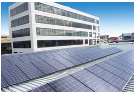
Solar panels, Hornsby Library roof
