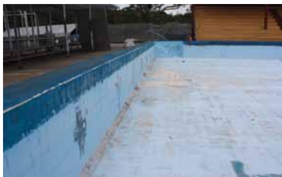
Hornsby Aquatic Centre was closed due to safety concerns
