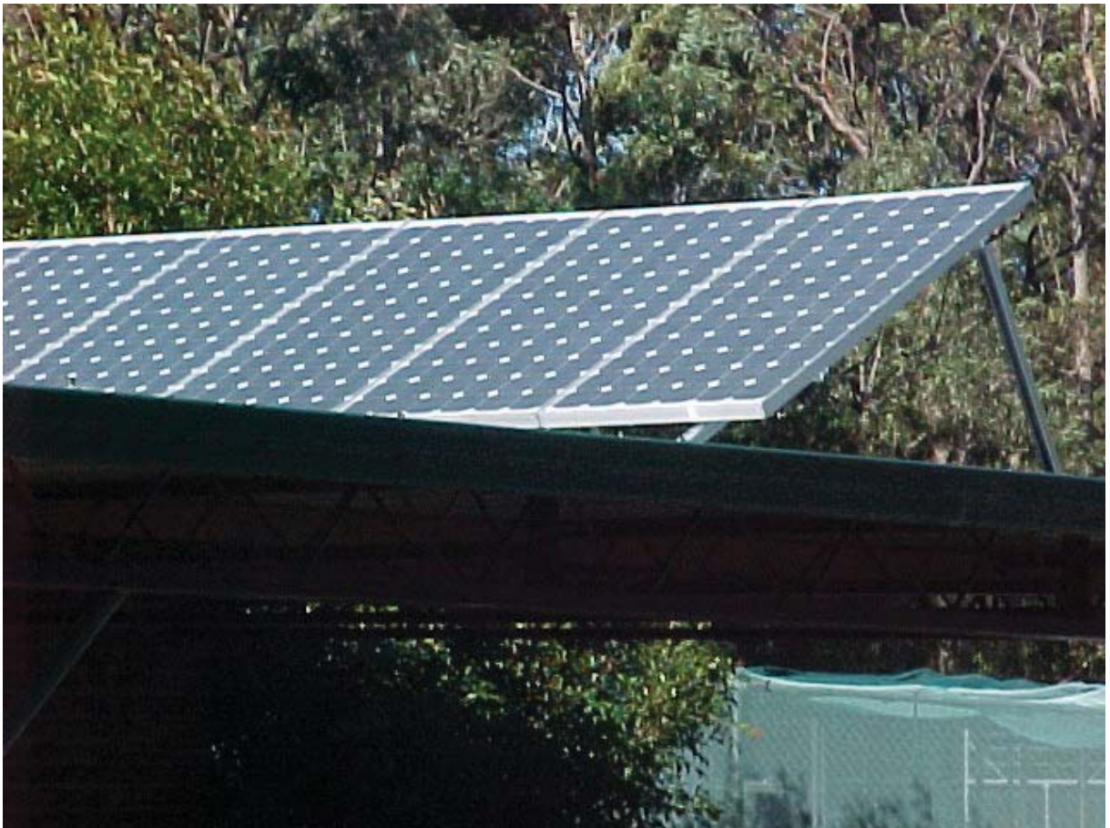
Solar panels on the Hornsby Community Nursery
