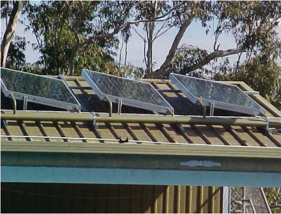
Solar collectors at Hornsby Aquatic Centre
