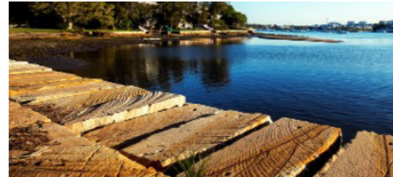
Stepped sandstone courses allow access to baths entry at varying water levels.
