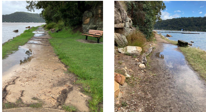
Existing inaccessible connection from Lower Mckell to Parsley Bay due to surface irregularities and ponding.
