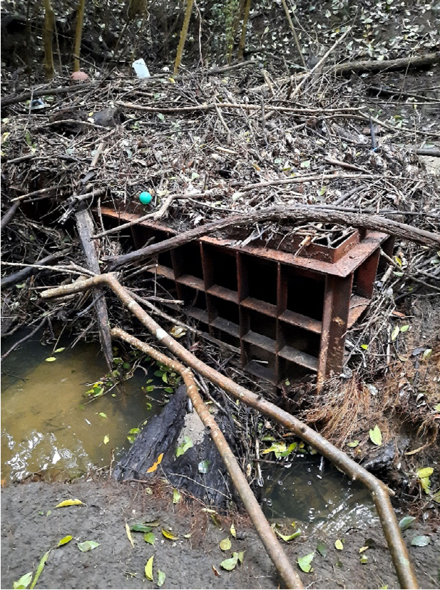
Photograph 5 Typical build up of debris and sediment following significant rainfall events
