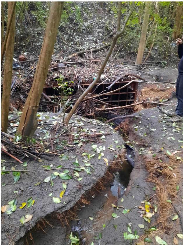
Photograph 4 Scouring and debris following the March 2021 storm
