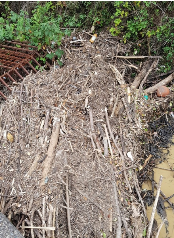
Photograph 3 Debris on the existing trash rack following the February 2020 storm
