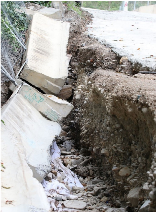
Photograph 1 Scouring and debris following the February 2020 storm
