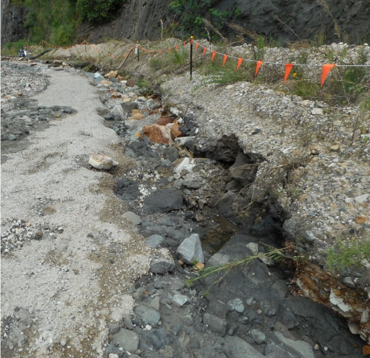
Photograph 2 Scouring following the February 2020 storm
